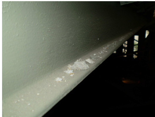
Figure 5. Chunks of asbestos is not removed by exhaust systems deposited on the metal structure.
