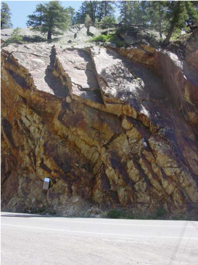
Fig. 3. Real road cut slope used in case study B. Image from Rockbench repository (Dataset 10a).
