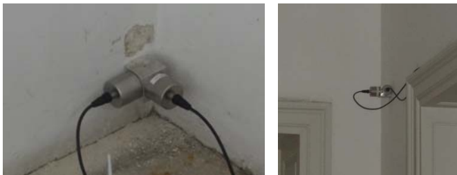
Fig. 11. Seismic accelerometers located in different positions on the building.
