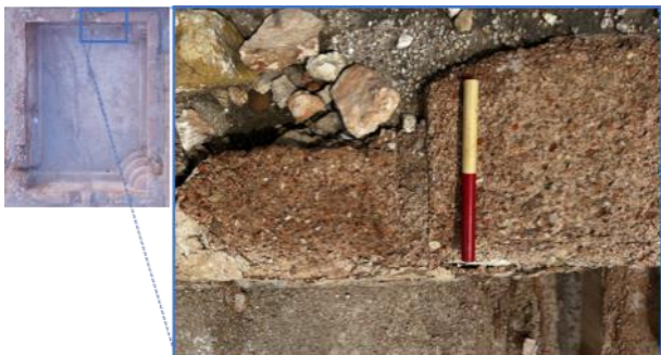
Figure 16: Photo of the north wall parapet. Semi-cylindrical hole 6cm in diameter filled with mortar is observed.
