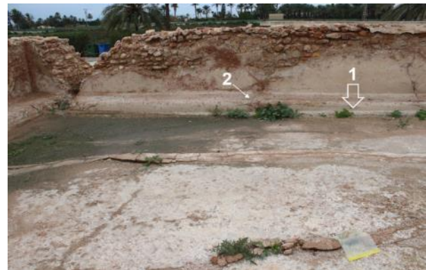
Figure 28: Appearance of the west face in the year 2022. Indicated as "1" is the arch-shaped discharge saddle. A recent crack is indicated as "2".
