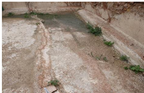
Figure 17: Appearance of the bottom of the natatio with cracks sealed with Opus Signinum creating a curved ledge. Photo taken in December 2022.
