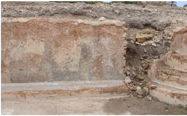
Figure 22: Appearance of the east wall next to the staircase in the southeast corner in 2022.
