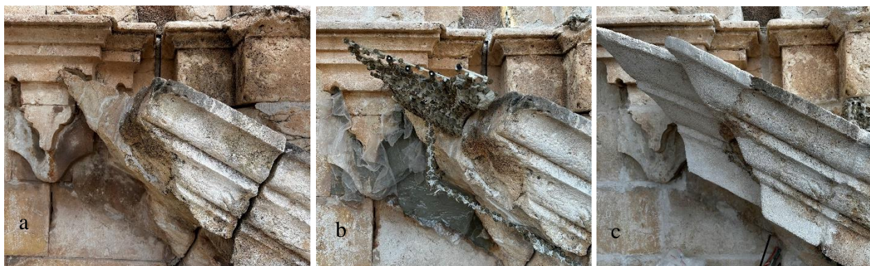
Figure 12. Different aspects of the restitution of volume using mortar with lightened core and light mortar. a) Missing area already consolidated while waiting to drill holes for anchoring. b) Appearance of the lightened core prepared to add mortar externally. c) Appearance with mortar already reintegrated, pending the application of glazing with lime water and pigments to blend the added area with the rest of the façade.
