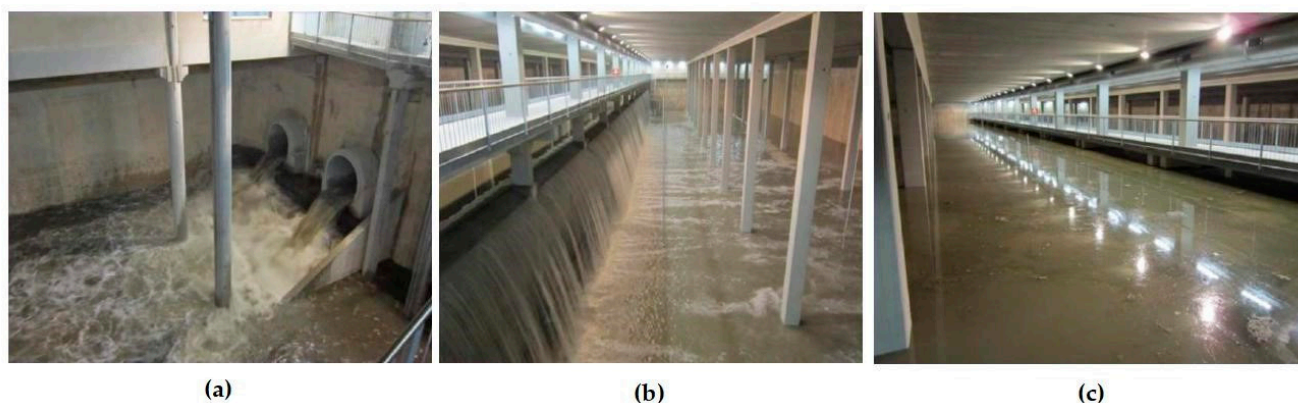
Figure 3. Filling process of the José Manuel Obrero Díez anti-DSU tank. (a) Tank filling through two 1.8 m diameter pipes; (b) Filling the tank; (c) Full tank. Source: AMEM. Own elaboration.
