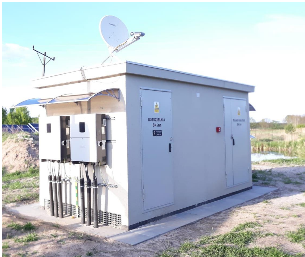
Image 75: Satellite Antenna mounted on the top of the transformer station. [own photo]
