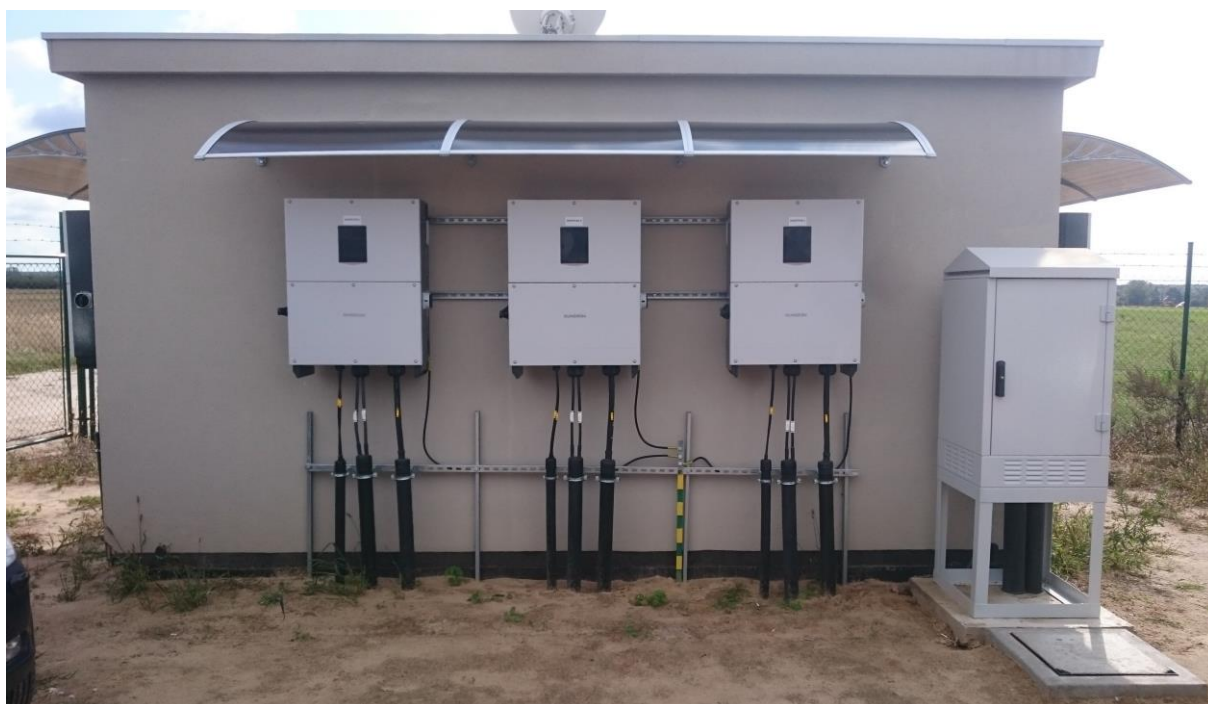
Image 53: CCTV cabinet next to a transformer station, at right side of the picture. [own photo]
