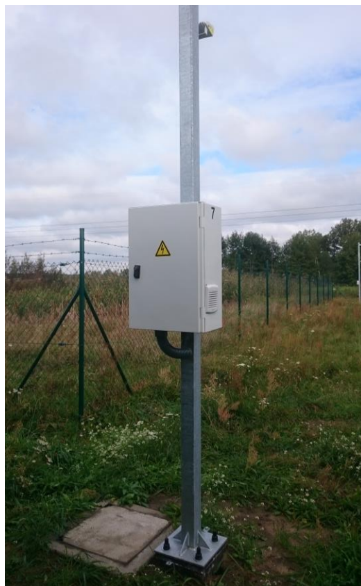
Image 57: CCTV AC3CON box. [company source]
