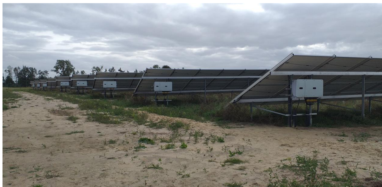
Image 30: Joint of 9 Huawei Inverters on a Lords photovoltaic farm. [own source]
