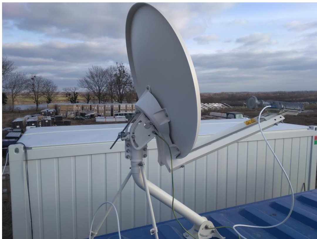
Image 76: Satellite antenna with rack and cabling. [own photo]
