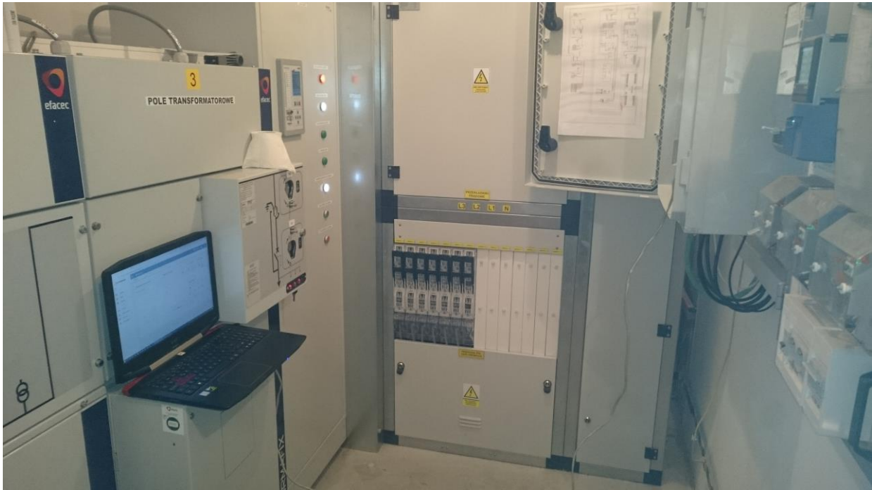
Image 23: Monitoring System inside the Transformer Station with a laptop connected. [own source]
