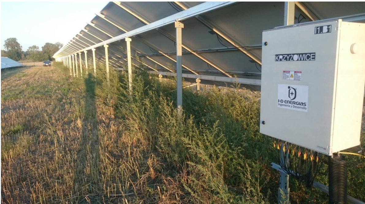
Image 11: String Combiner Box mounted over photovoltaic structure. [own source]
