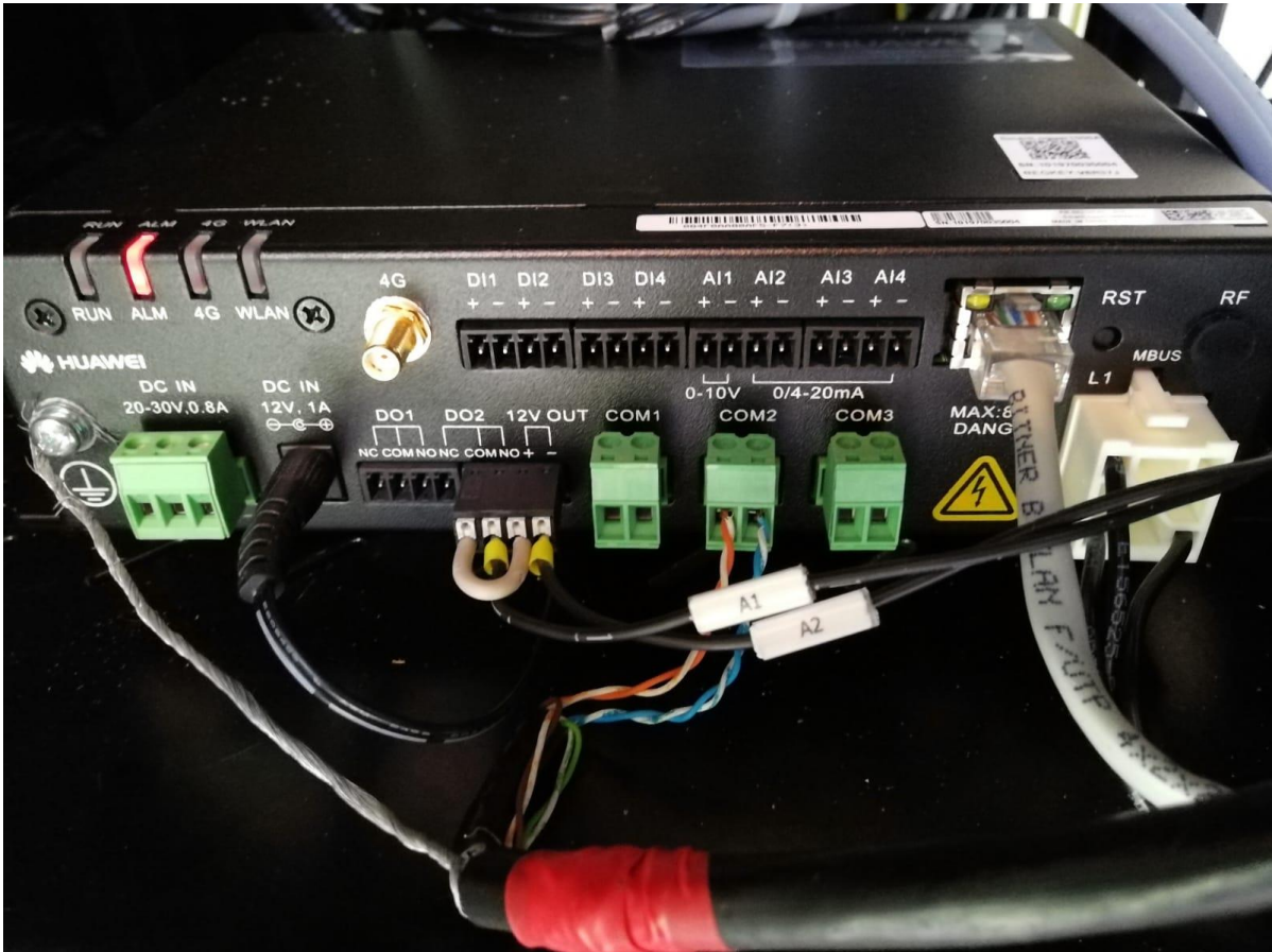
Image 38: Rear view picture of Huawei’s Smartlogger. [own photo]
