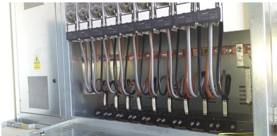
Image 26: 9-inverter busbar architecture inside the trafo station. [own source]
