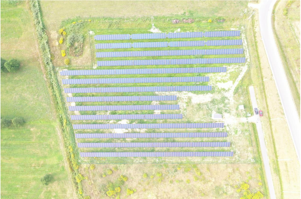
Image 6: Piaski 1 MW PV farm photo taken with a drone (2). [own photo]
