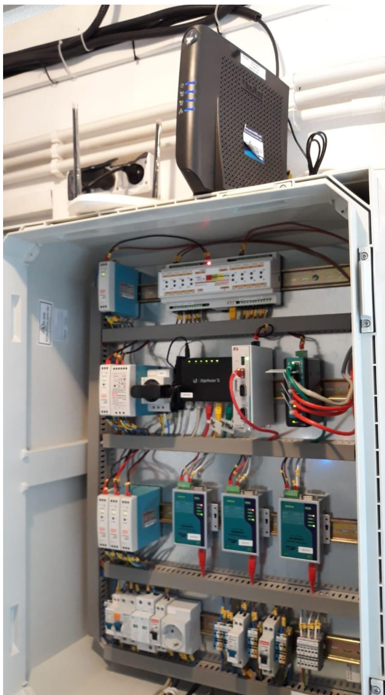
Image 74: Satellite Modem and Router already connected to the monitoring cabinet, inside transformer station. [own photo]
