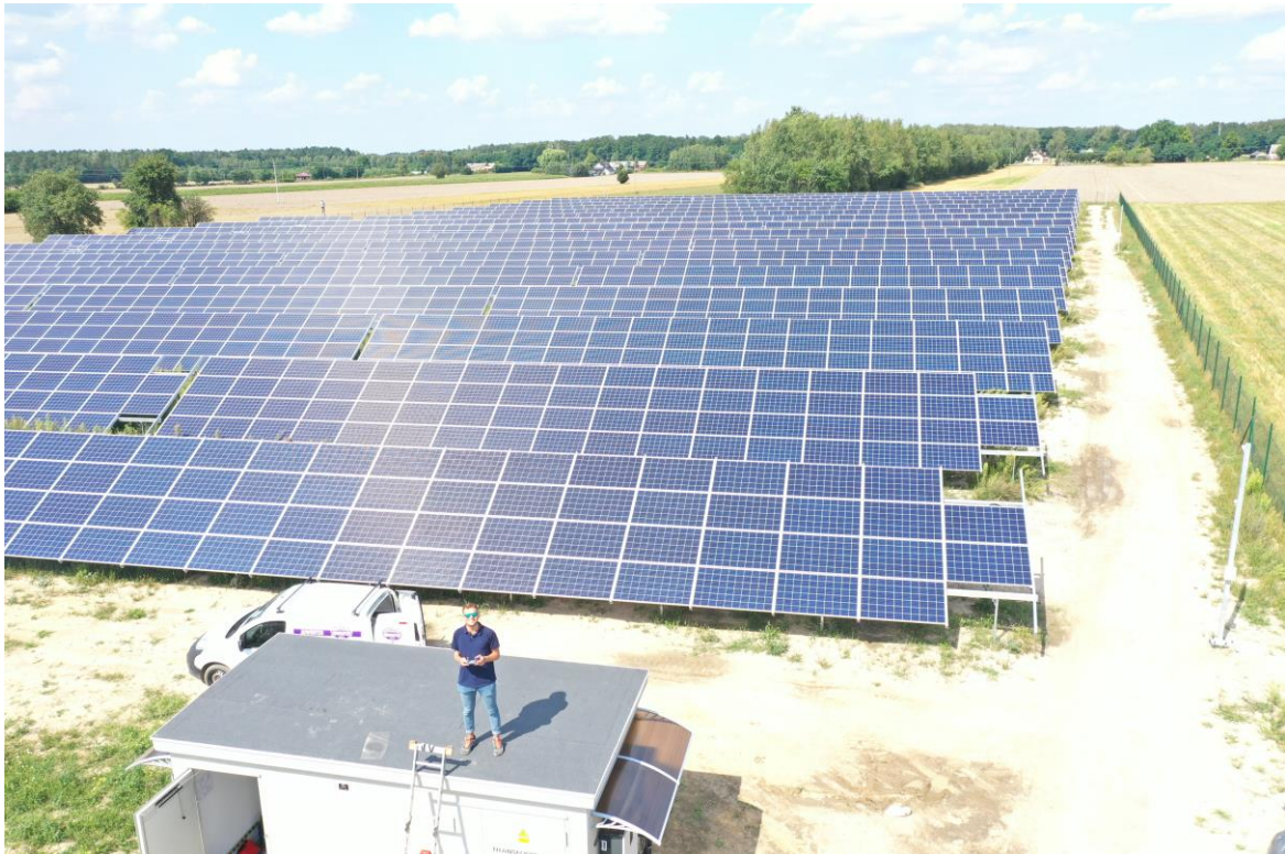
Image 5: Piaski 1 MW PV farm photo taken with a drone (1). [own photo]
