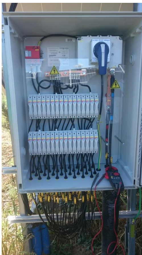
Image 15: Interior of String Combiner Box. [own photo]
