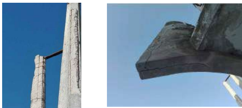
Figure 3. Detail of damages observed on the r.c. structures on the Church of Santa Maria Assunta bell tower.
