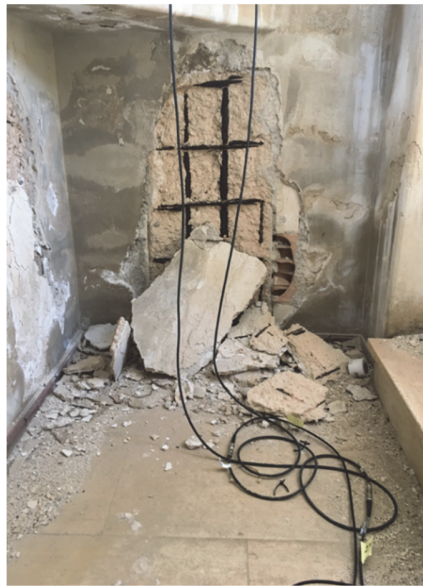
Figure 14. Corrosion effects detected on the bell chamber at a quote of 40 m from the ground level.
