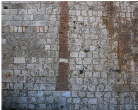
Fig. 7- Rectified photography the shows a part of the west flank of the bastion of Santa Croce . We can observe the original materials adopted in the sixteenth century and characterized by a unique dimension
