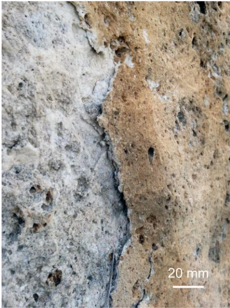
Fig. 8- Compact limestone ashlar of Santa Croce's wall facade, with evident exfoliation and pitting processes and detachment of flake with thickness about of 5 mm
