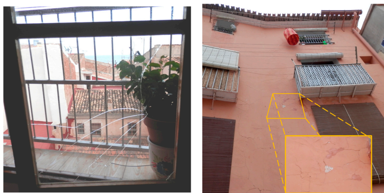
Figure 25. Some damages detected after tests.
