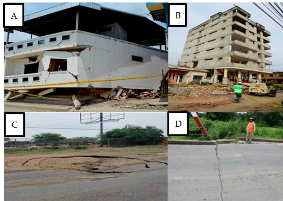
Figure 6. Evidence of the Pedernales earthquake on 16 April 2016, in the city of Chone with affection in buildings, houses and in the southern zone in the urban area presence of liquefaction. (A) Structural failure in the building caused by construction flaws; (B) non-uniform settlement in the foundation; (C) settlement on soft ground produced by liquefaction effects; (D) deformations or decoupling in pavement structures.
