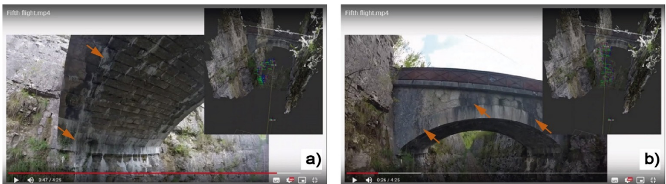
Figure 7. Mineral precipitations in the joints (a) and lichens growth (b) of bridge 1 pointed out by orange arrows. Note the geolocation image of the drone in the upper right corner of both frames, which allows the engineer to know the position of the displayed image in real time during the analysis of the videos.
