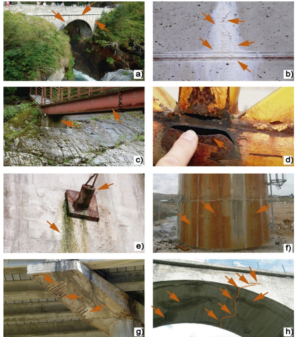
Figure 3. Some common damages that can affect bridges: (a) efflorescences on a masonry bridge in Caunterets, France; (b) efflorescences and crack in a reinforced concrete wall; (c) lichen growth in abutment and corrosion of a steel bridge beam in Lanuza, Spain; (d) crack and corrosion in steel truss handrail in Alcoy, Spain; (e) lichen growth caused by excessive humidity and corrosion in cable anchor plate in abutment in Benidorm, Spain; (f) rust stains in a surge chamber; (g) concrete spalling due to corrosion of steel reinforcement in a bridge in Petrer, Spain; (h) transverse cracks on reinforced concrete arch of bridge in Alcoy, Spain.
