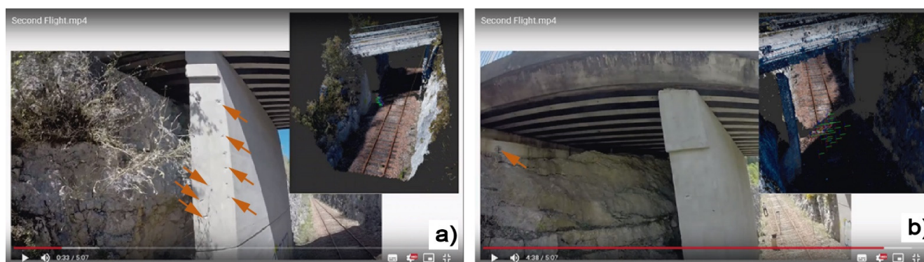
Figure 8. Concrete spalling due to reinforcement corrosion in column P1 (a) and abutment A1 (b) in bridge 2.
