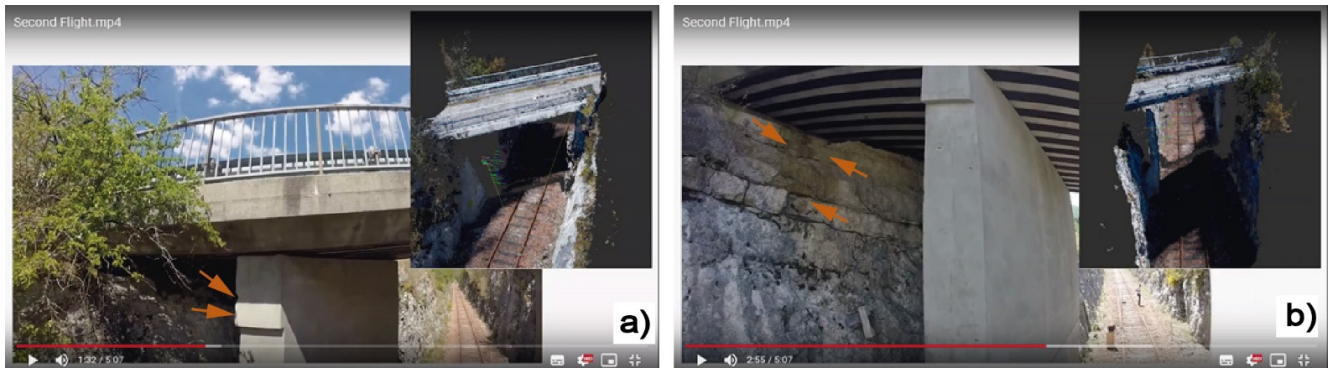
Figure 9. Failures caused by impacts (a) and lichens growth on abutments (b) in bridge 2.
